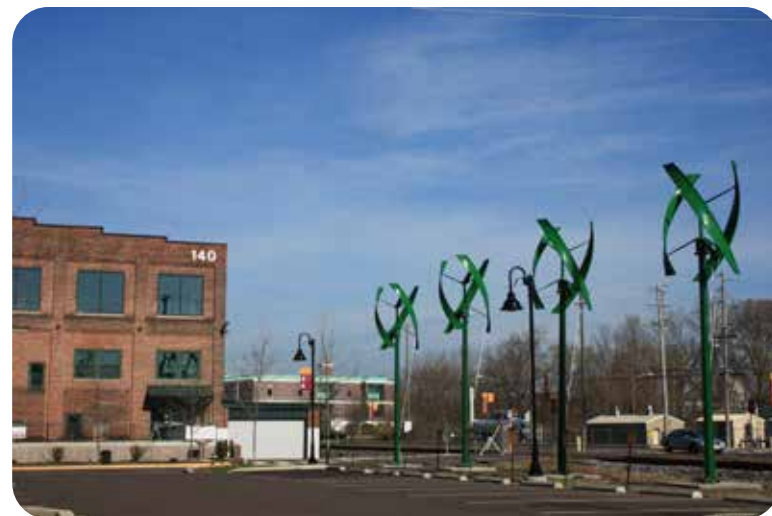
WITH A RANGE OF DESIGN AND SCALE OPTIONS, SMALL WIND ENERGY SYSTEMS CAN BE INTEGRATED INTO A VARIETY OF SITES. THESE VERTICAL AXIS WIND TURBINES POWER THE LED LIGHTS OF THE PARKING LOT AT MONTGOMERY COUNTY COMMUNITY COLLEGE-WEST CAMPUS IN POTTSTOWN.
