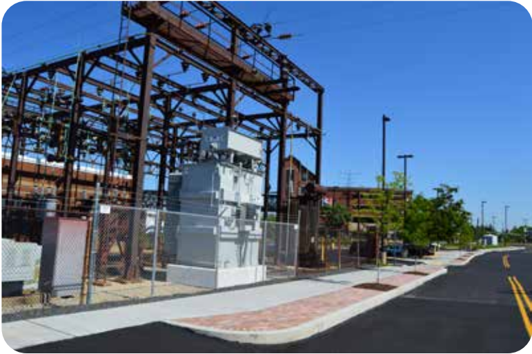
LANSDALE IS ONE OF ONLY TWO MUNICIPALITIES IN MONTGOMERY COUNTY WHICH HAS ITS OWN ELECTRIC DEPARTMENT.
